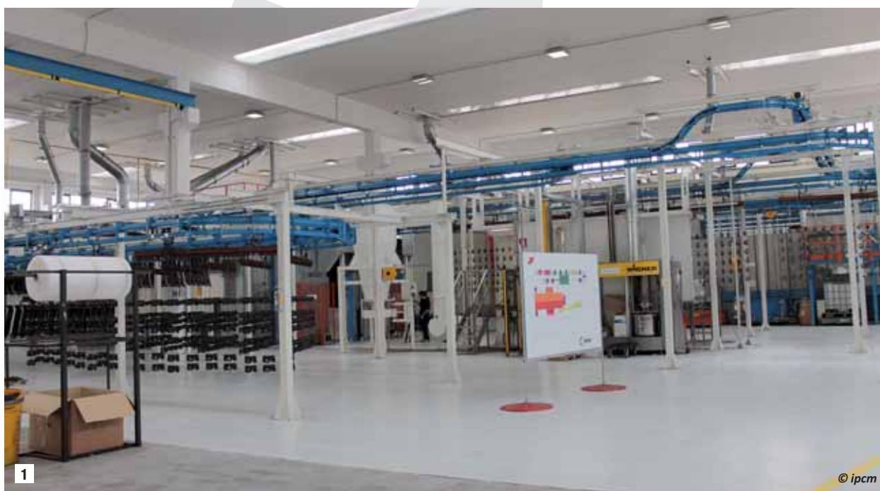
1 An overview of Caroni Spa's new paint shop, following the decision to insource all the coating operations.
