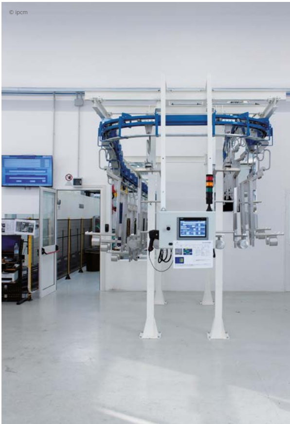
The loading area of the pre-treatment tunnel's overhead conveyor.
