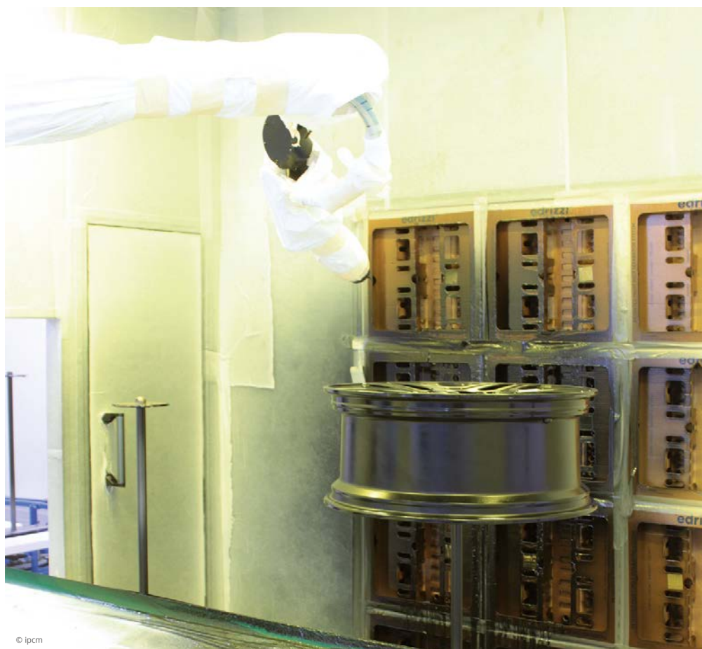
The CMA Robotics robots’ control units outside the booths.
